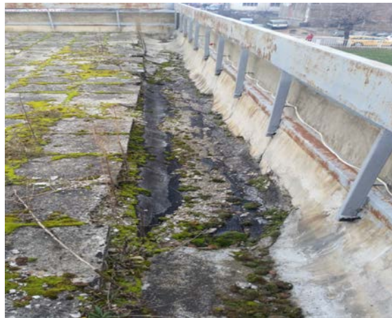
*Damaged slope layer in the gutter detail
